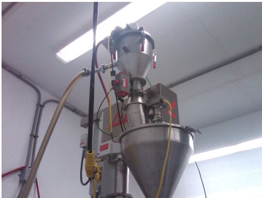
VAC-U-MAX custom pneumatic conveying system above filling machine at Nutriom plant.
